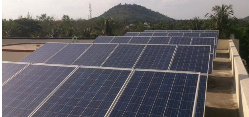
Figure 2. Picture of 18 kW PV plant at Ranipet (PV Plant 2)
