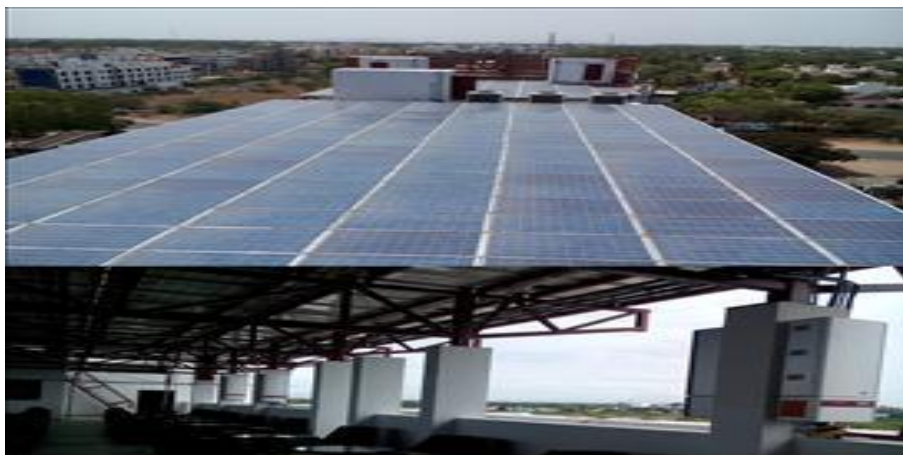
Figure 1. Picture of 84 kW PV plant at Tirunelveli (PV Plant 1)
