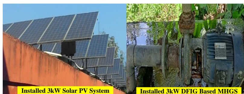
Figure 3. Installed renewable generation system
