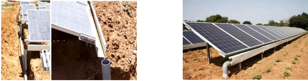
Figure 4. Rain water harvesting system on AgropV [23]–[25]
