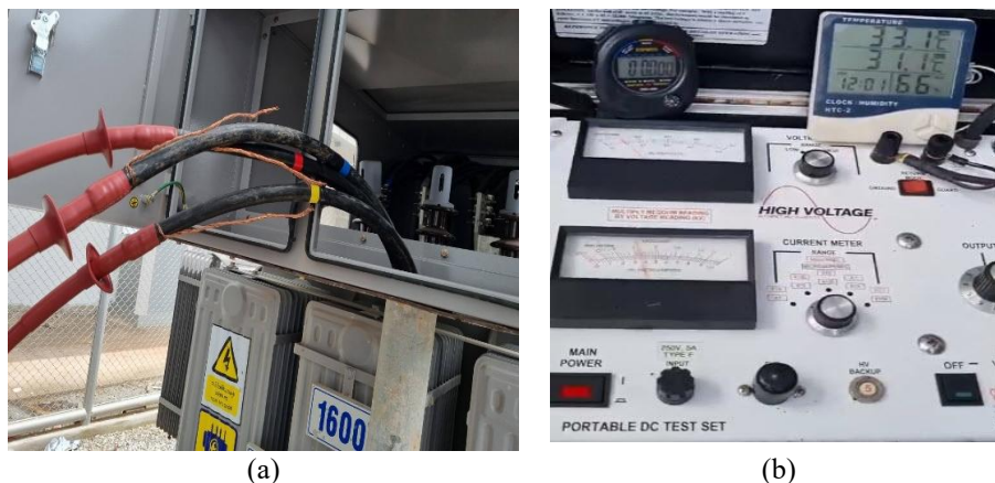
Figure 5. Equipment used for insulation resistance testing: (a) termination kit for insulation resistance testing and (b) portable DC test set
